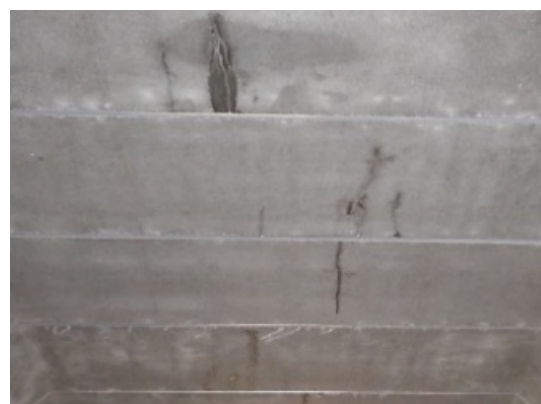
Fig.1 Water leakage from joint gap
